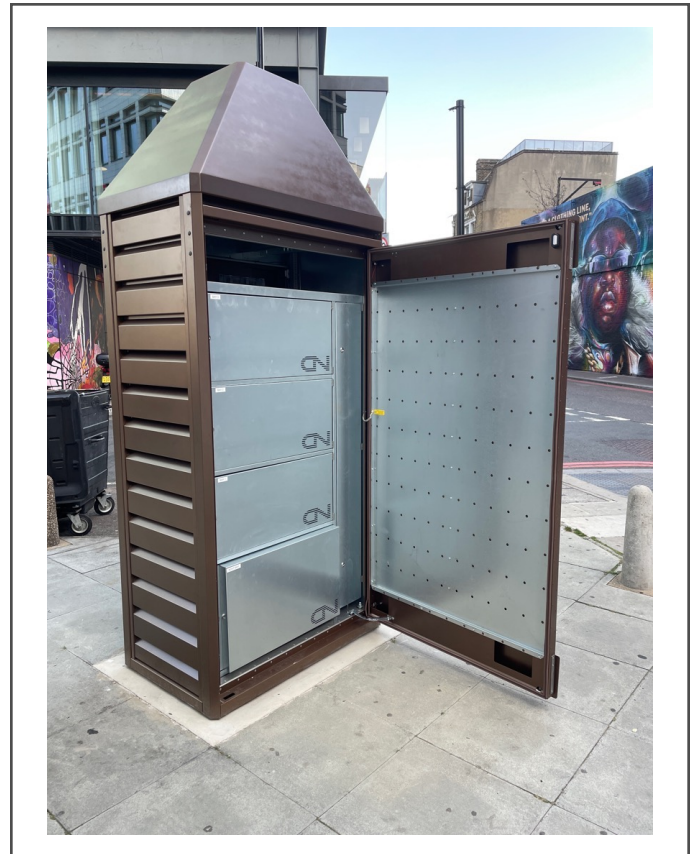
Figure 1. Street Arc enclosure from CIN.
